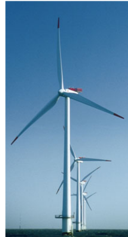
Offshore wind farm
