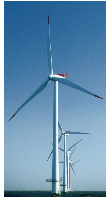
Offshore wind farm
